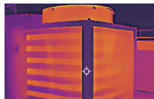
HVAC Leak Detection
